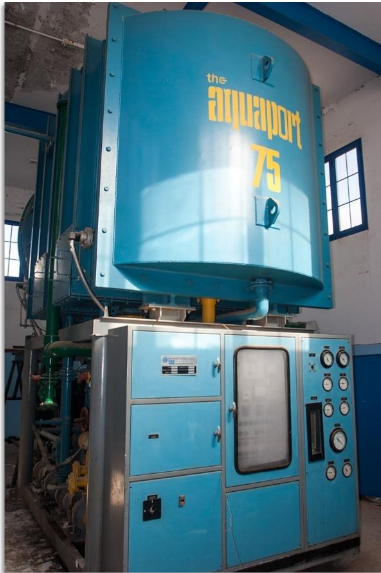
Potabilizadora VC IDE 380v – 50cv 1977
